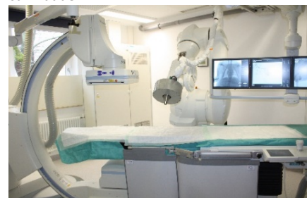
Installation of a TX 200 high-performance 6-arm robot from Stäubli in SEON's animal operating room for precise control and positioning of the magnetic field.
